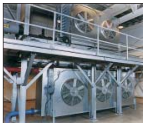
EVAPORATOR TEST STAND
